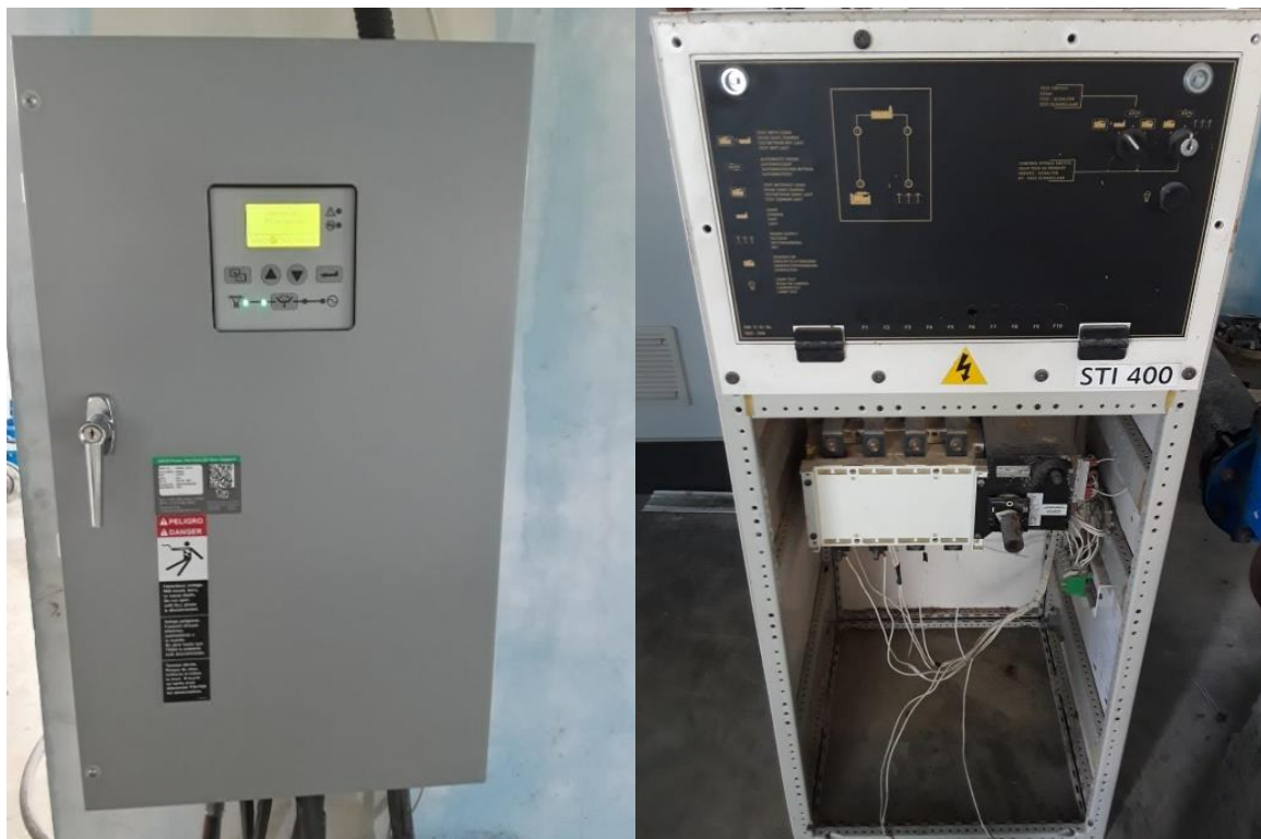
Image 1: Left: New ATS installed, Right: Previous Manual Transfer Switch.
