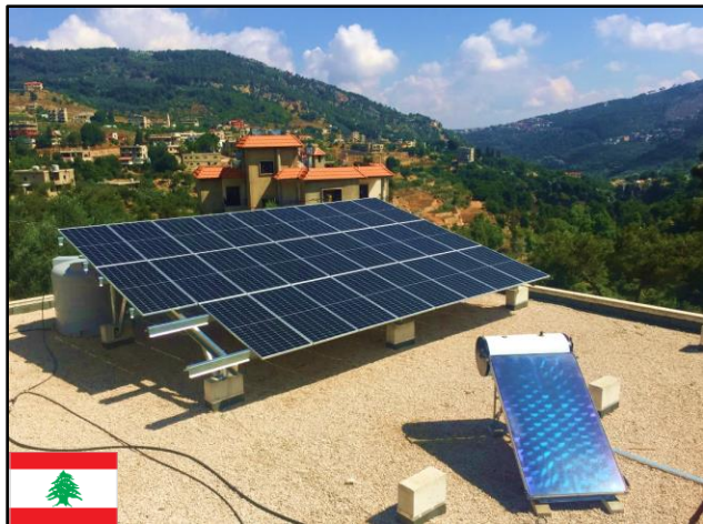
25 kWp on-grid solar PV system with a 90-kWh storage capacity and a 200-liter solar water heating (SWH) system for the agro-food and beekeepers cooperatives' building in Akkar Al-Atika, Akkar, Lebanon.
