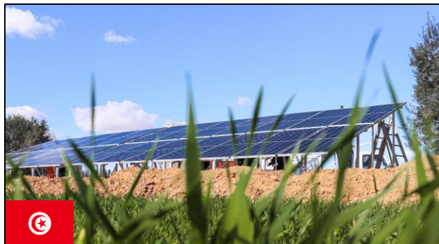
10.4 kWp solar PV water pumping system for Mr. Abdallah Ben Mansour's farm in Chorbane, Mahdia, Tunisia.
