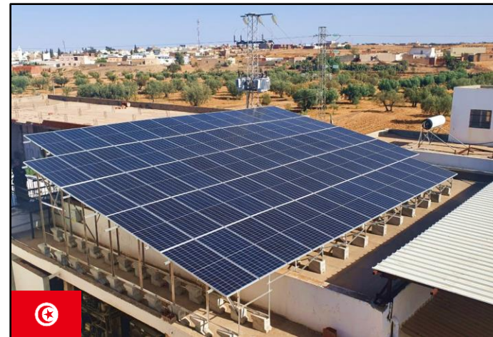
65.5 kWp medium-voltage on-grid solar PV system for the mutual agricultural services company "El-Faouz" in Mahdia, Tunisia.
