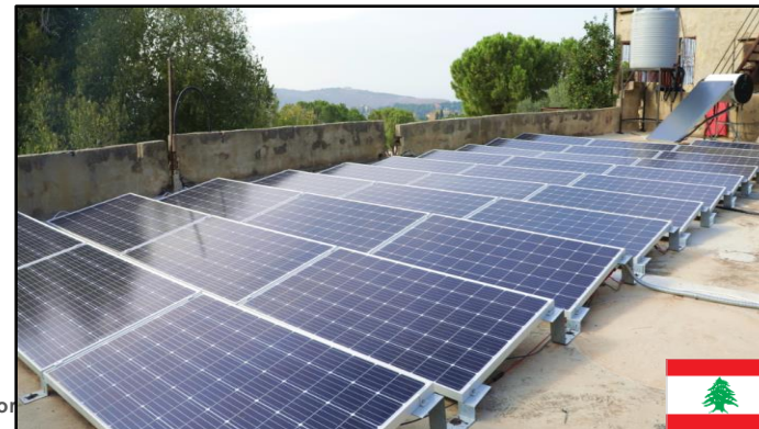
10 kWp on-grid solar PV system with an 18-kWh storage capacity and a 200-liter SWH system for the "Live Akkar" Organization – Sewing and Embroidery Workshop in Chaqdouf, Akkar, Lebanon.
