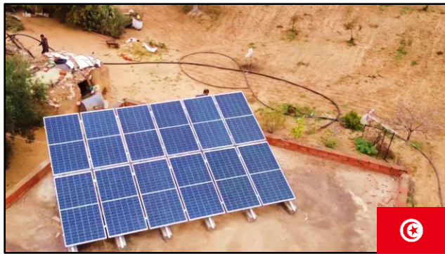
4.8 kWp solar photovoltaic (PV) water pumping system for Ms. Fethia Bougtif's farm in Chorbane, Mahdia, Tunisia.
